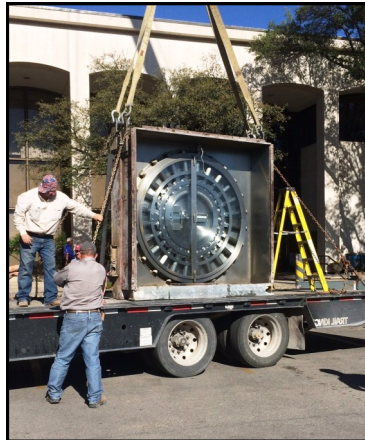
Skilled crew prepare vault door for transport to newly constructed bank building on Concho Avenue.
